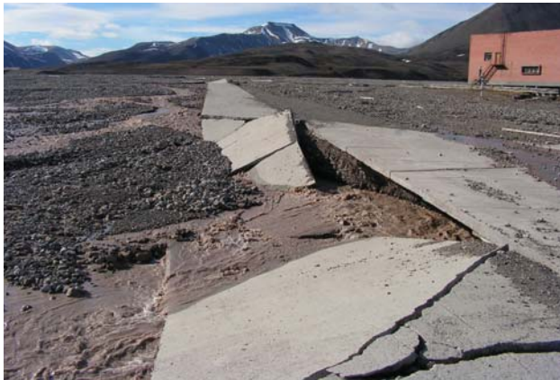
Picture 6.1 Street damaged by the Bertilriver in Pyramiden
