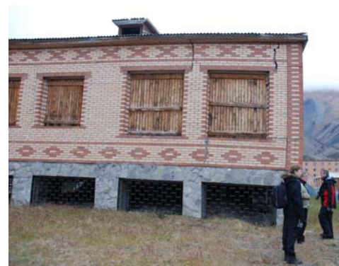
Picture 8.5 Kindergarden in Pyramiden with differential settlements
