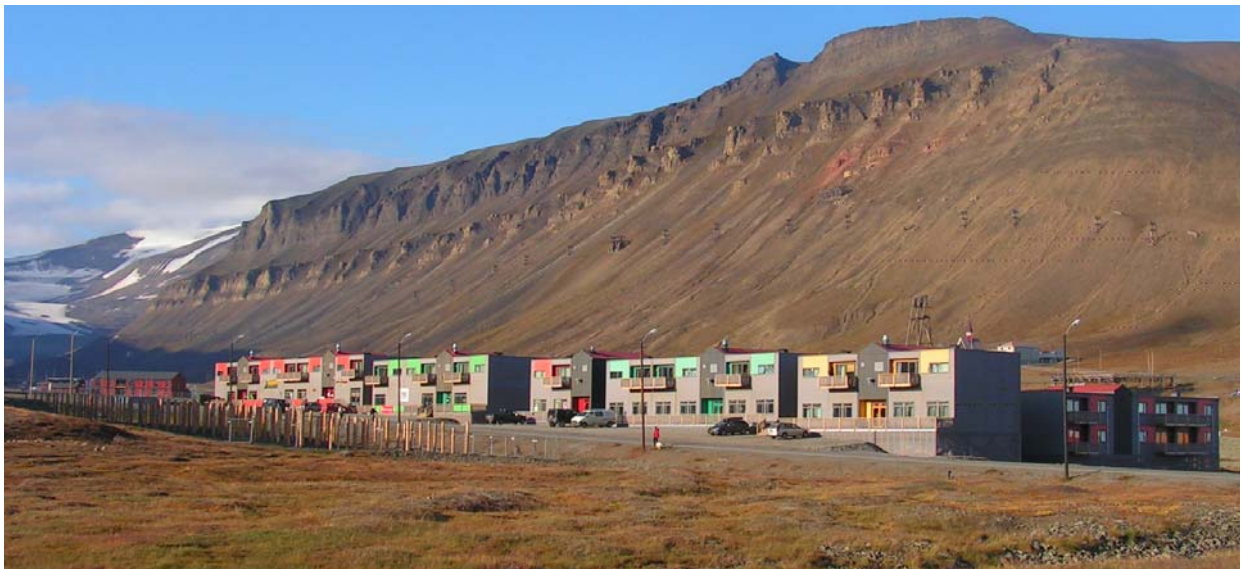
Picture 9.1 New building site with wooden piles already in the ground in Longyearbyen
