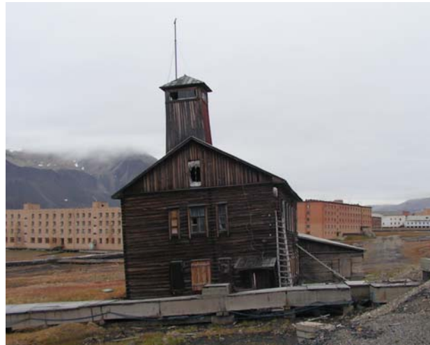
Picture 8.2 Lateral creep dips the firehouse in Pyramiden
