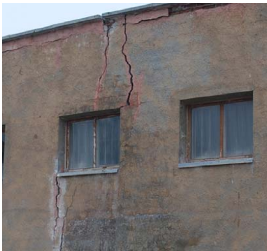
Picture 8.1 Cracks due to primary creep in Pyramiden
